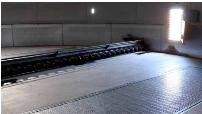
IN-FLOOR AERATION SYSTEM
